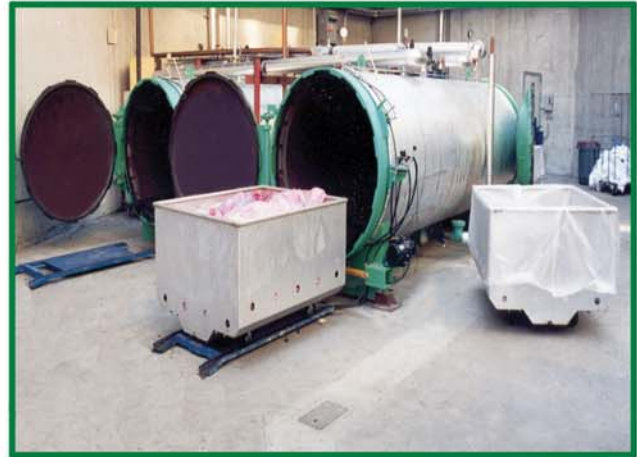
These AS515 units with optional Double Doors installed at a large regional California hospital meet the demand for reliable and dependable waste equipment.
