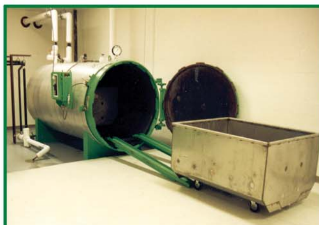
Equipped with optional cart ramp this AS510 installed at a Regional medical center allows carts to be easily loaded into sterilizer.
