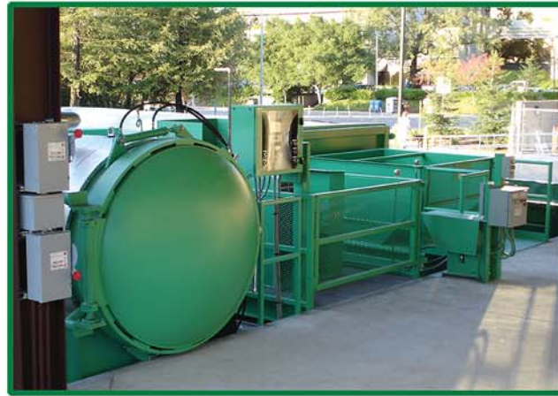
AS510 with vacuum and touch screen controller installed at dock with self-contained compactor for waste and stationary compactor for OCC.
