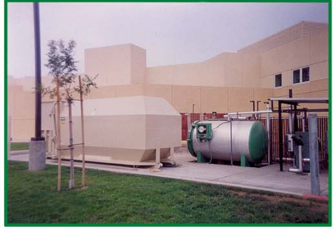
Installed with a self-contained compactor at a prestigious Western Medical facility this AS510 allows EVS to manage their solid and medical waste.
